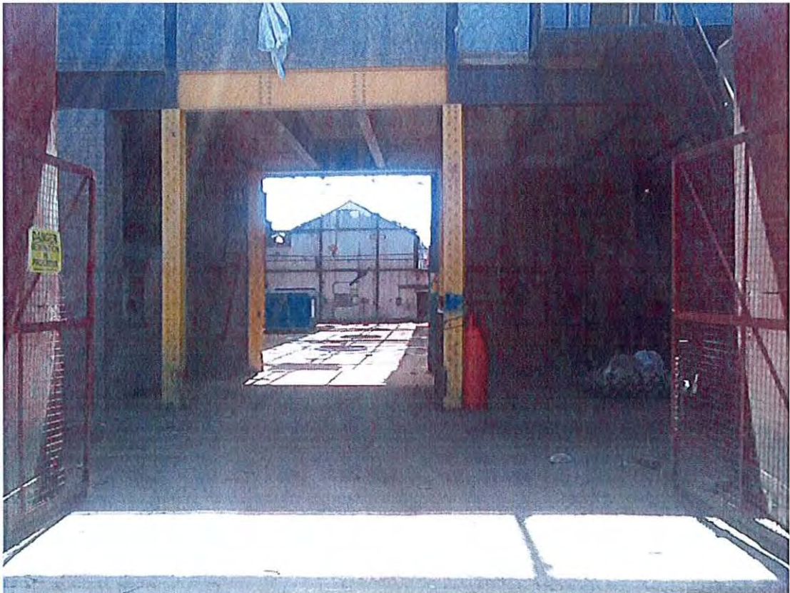
Figure 6 A view inside the existing building on the eastern part of the site from the NE corner.
