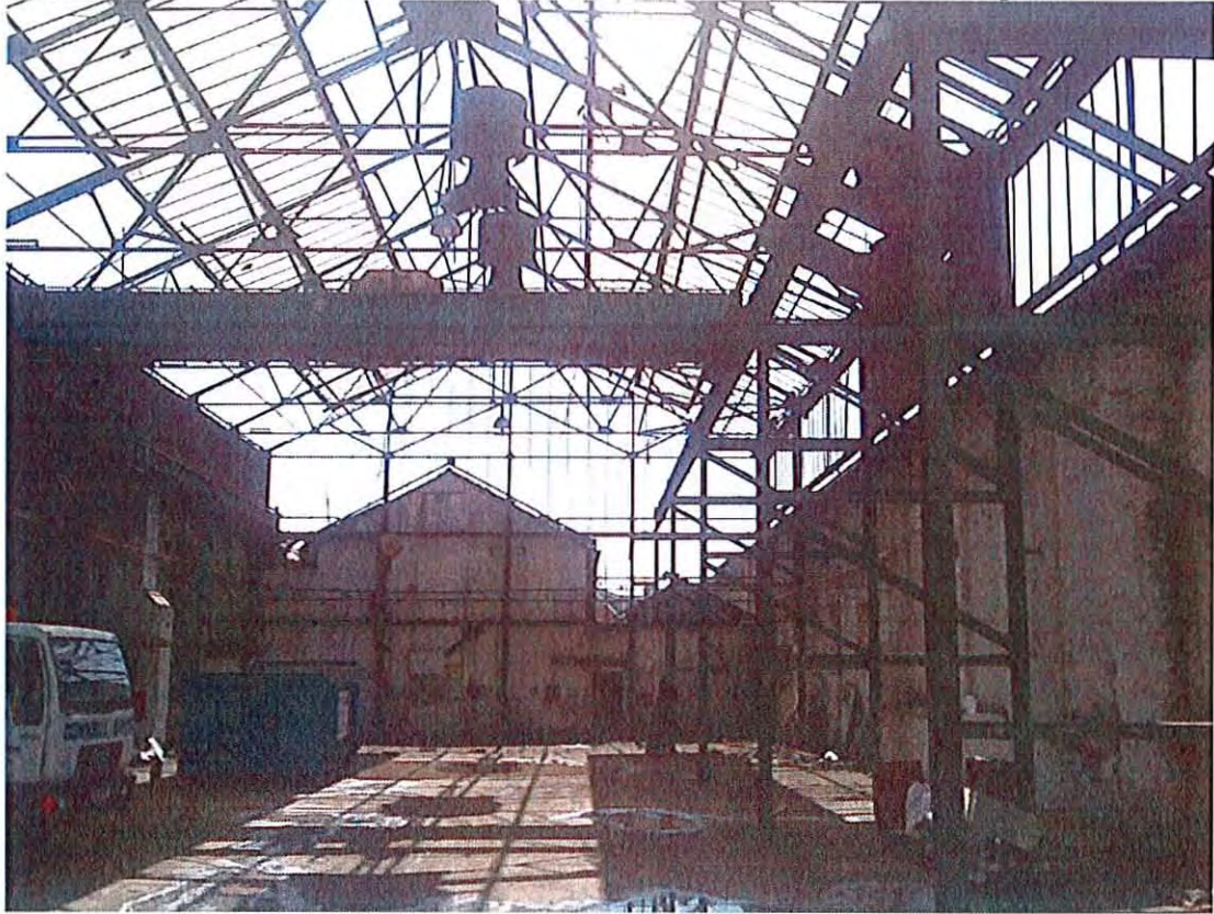
Figure 15 A view to the south from inside the existing eastern building on site.
